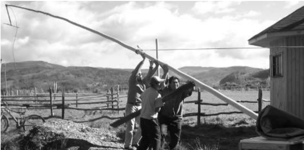
Chile. Raising the aerial at WACC-supported indigenous Radio We Keche shortly before beginning to broadcast.
